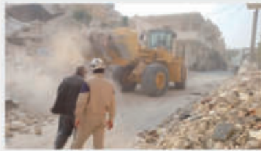
Emergency responders clear rubble with Syria Regional Program-provided heavy machinery following a regime attack in Maaret Nauman, Idlib, in November 2024.
